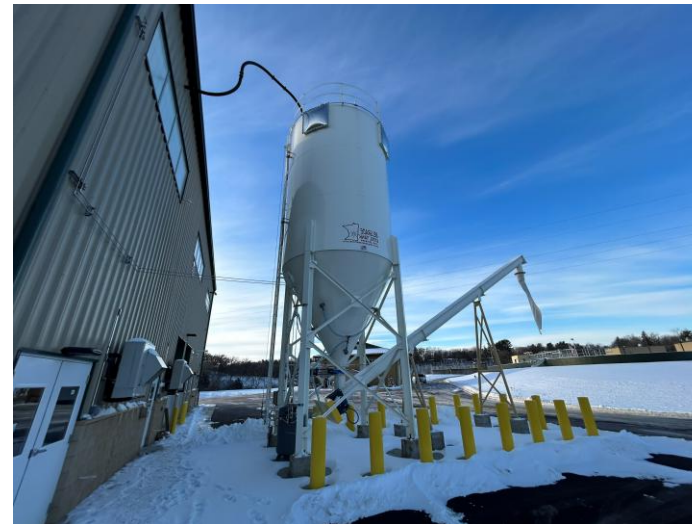
Dried biosolids storage silo (River Falls, WI)
