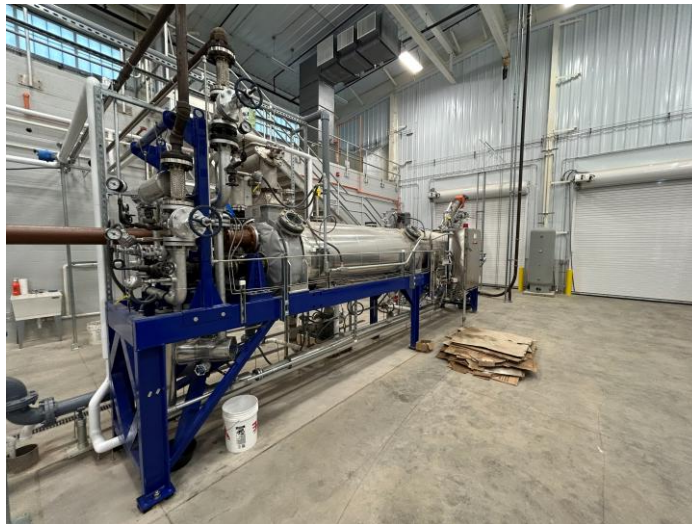
Biosolids dryer (River Falls, WI)
