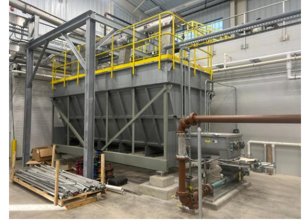
Dewatered cake hopper (River Falls, WI)
