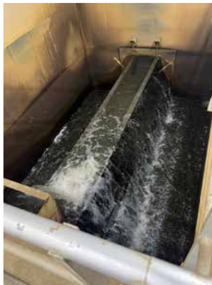
Sand filters at the City of Platteville WRRF prior to upgrades
