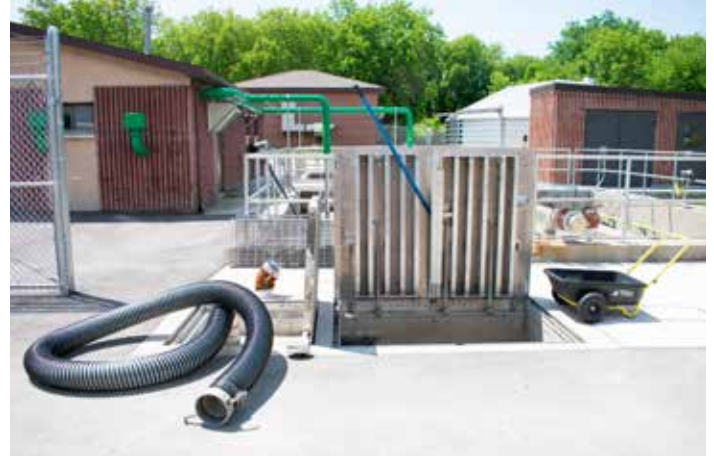
New hauled waste receiving station
