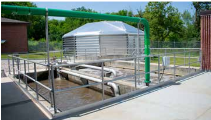
Anaerobic tank and aerobic basin
