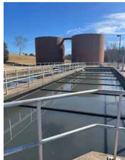
Primary clarifier at the City of Platteville WRRF (Trickling filters in background)
