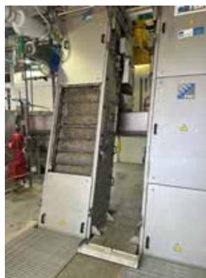
Mechanical fine screens
