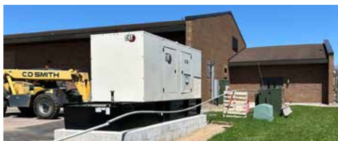
New diesel generator
