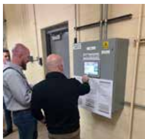
Aerzen blower control panel
