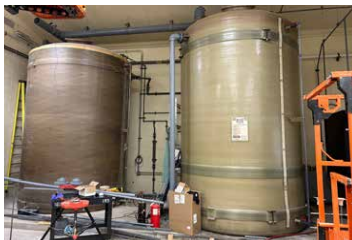
Existing phosphorus removal chemical tank on left, new PRC tank on right. Used to use Alum, now use PAC.
