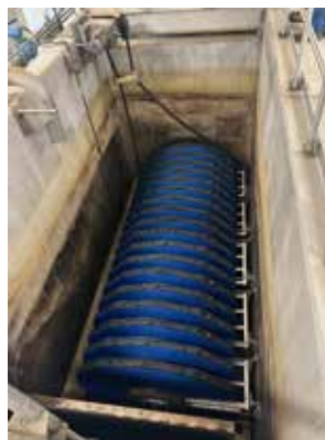
Low level phosphorus tertiary filters
