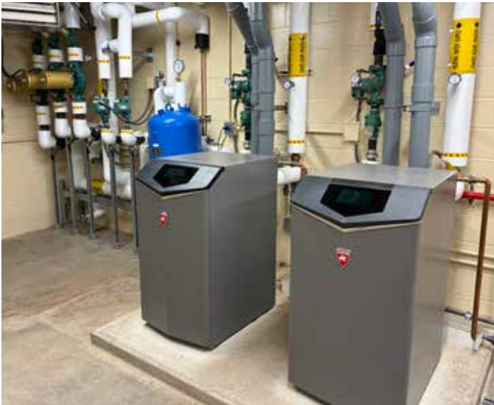
New building heat boilers
